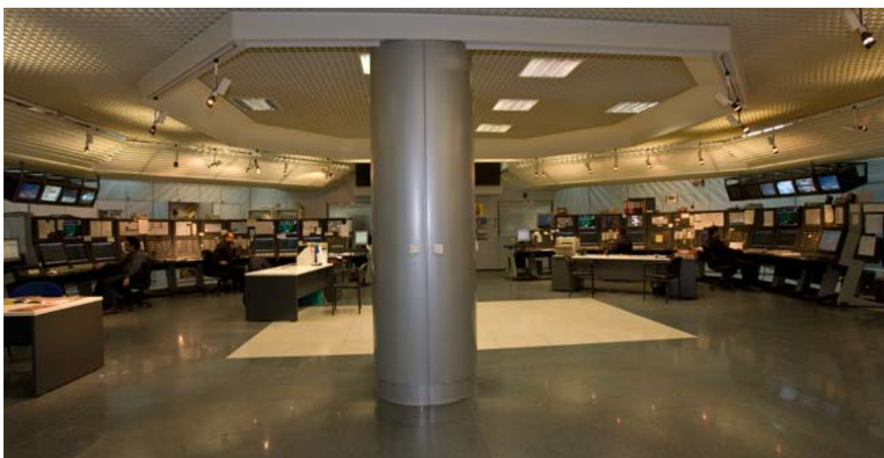
Control Room - Thessaloniki Refinery
