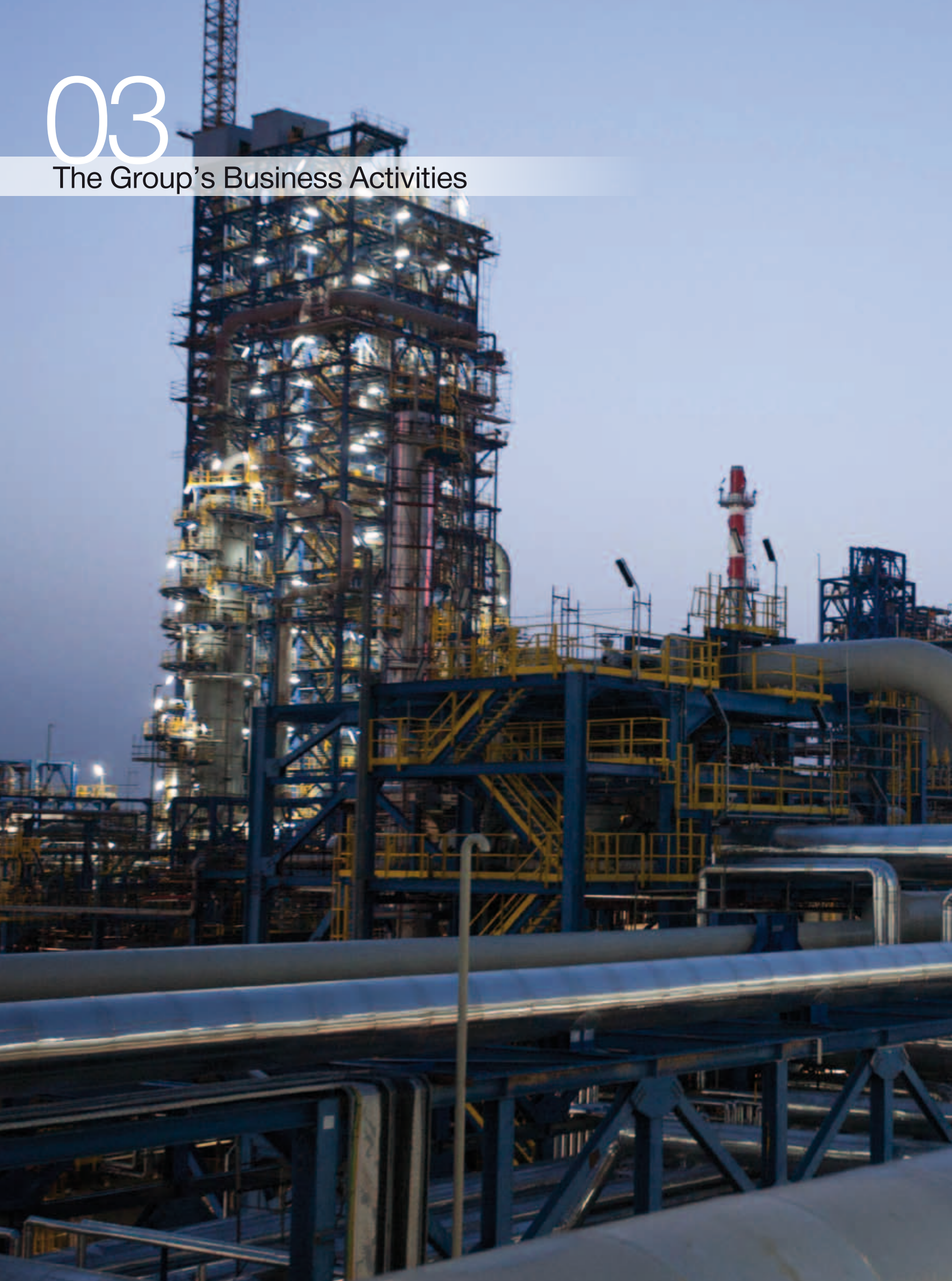
Unit-32 - Flexicoker Reactor - Fractionator & Steam SuperHeater - Elefsina Refinery
